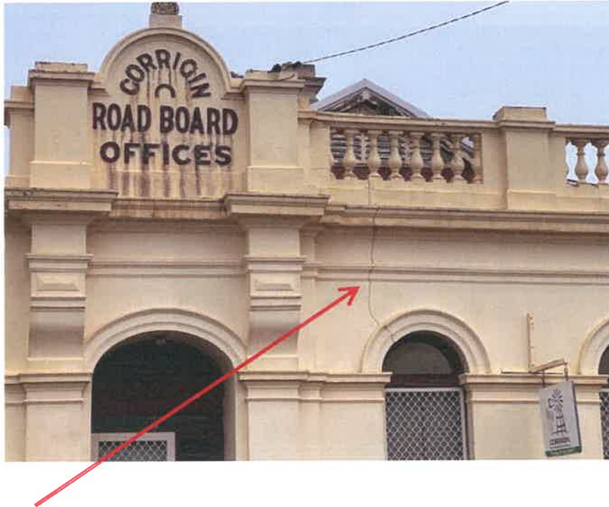
Major cracks to be repaired
