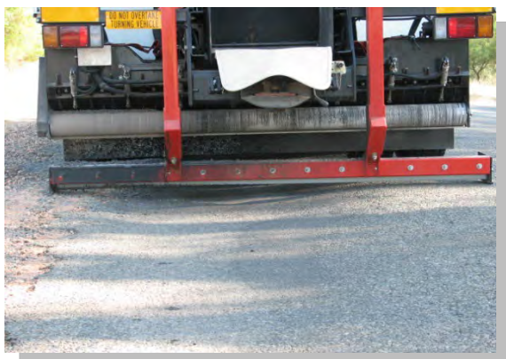
Before wheel rutting repairs
