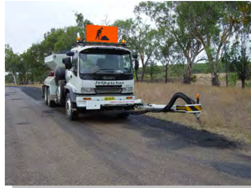
Jetmaster® boom fully extended during repair job. Movement is restricted to the right for safety.
